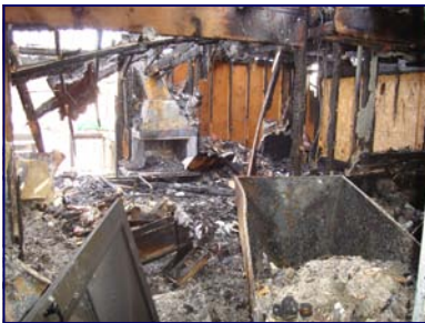
The family room after the fire
